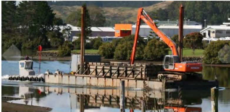
Example of a flat top spudded hopper barge, with an excavator onboard. The excavator digs material and places onto the same barge the excavator is mounted on.
