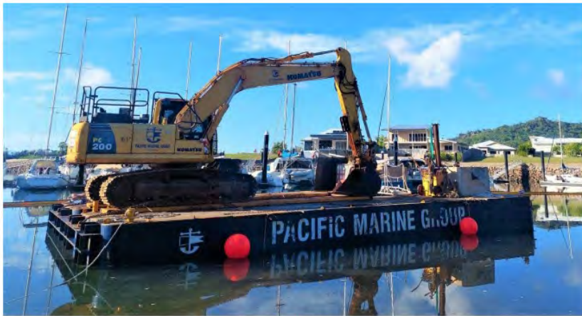
The secondary dredge platform, with 20t Excavator, dredging in Nelly Bay Harbour
